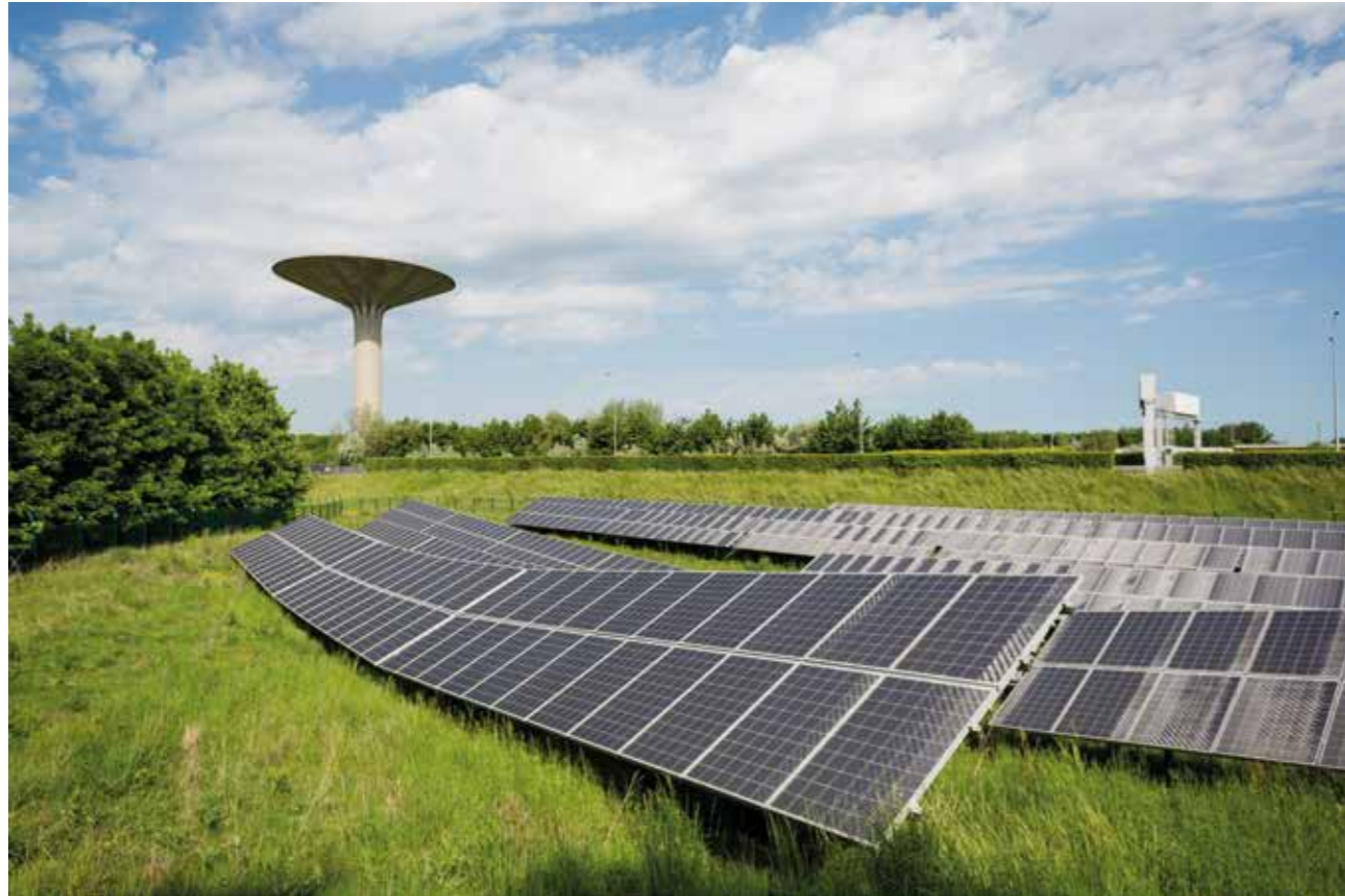
Solar farm - North Environmental and Sustainable Development Resource Centre, Paris-Charles de Gaulle Airport
